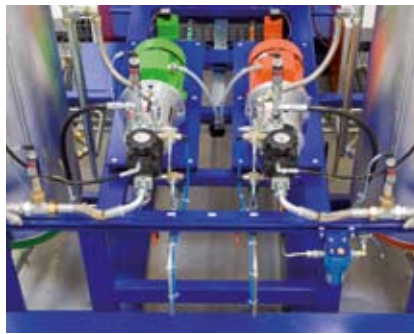
Pump assemblies (isocyanate side with high pressure filter), manual calibration valves
